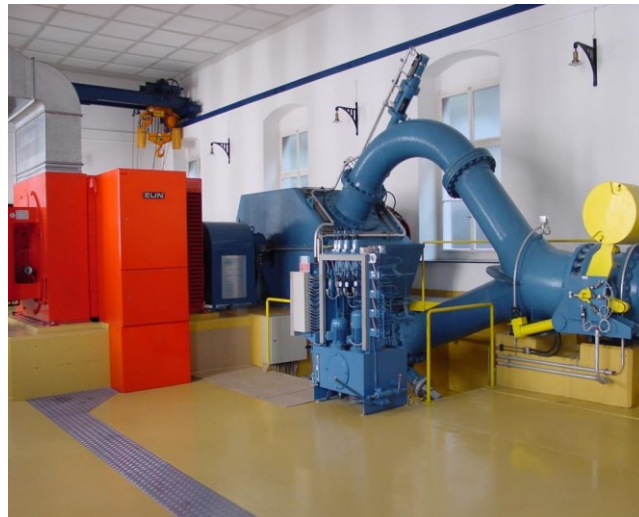
KW Felsen 1 (1993, 1'477 kW)
